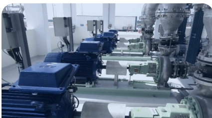
Pump motors and pipework
