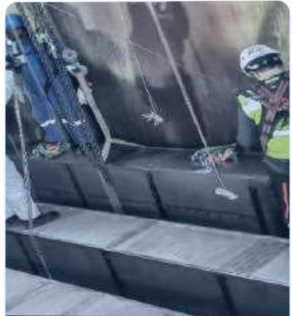
Bypass stack silencer baffle
