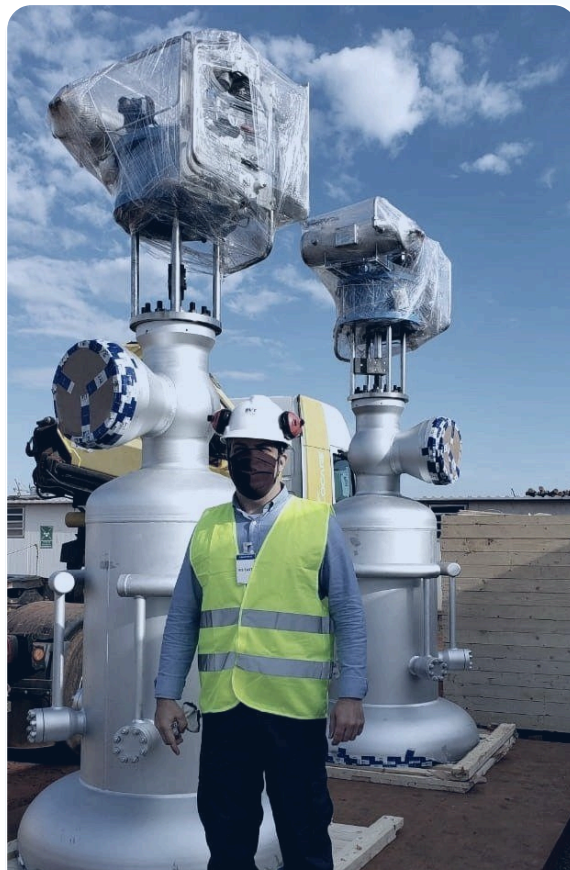
Bypass valve installed on site
